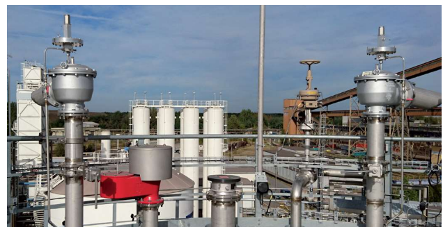
Cryogenic Storage Tank
